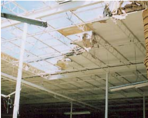
Wind damage from F2 tornado / Dade County March 27, 2003
